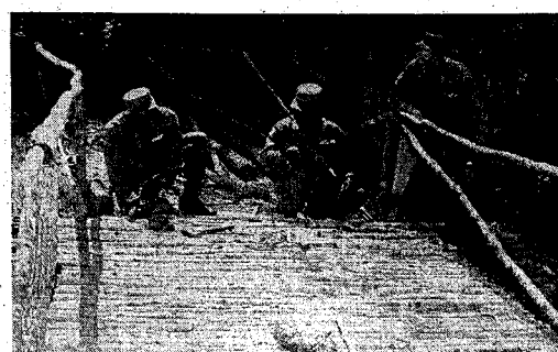
BRIDGEWORK... The final touches are being put on this bridge in the Engineer Training area by members of Company A, 78th Engineer (C) Battalion. Left to right are Cpl. Sammy Wilson, Pvt. John McQueen, and Cpl. William Steen.
